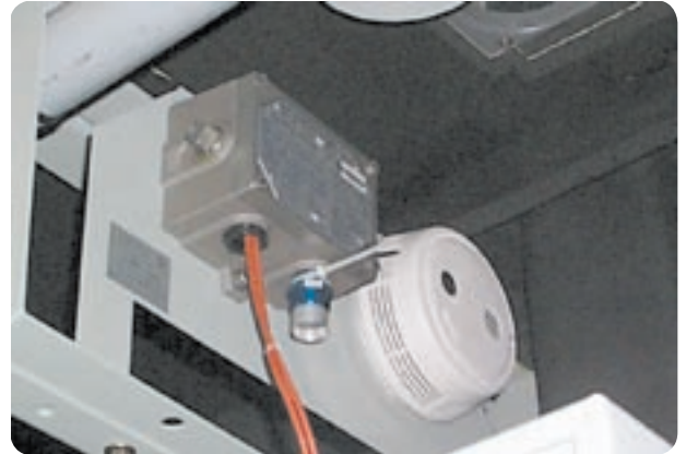
Hydrogen and smoke detectors.
