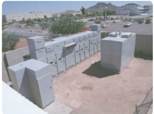
Medium-voltage PureWave UPS System.
