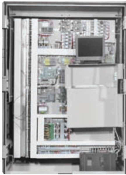
System control and system monitor.
