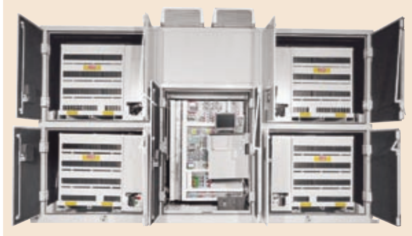
Energy storage container rated 2500 kVA.
